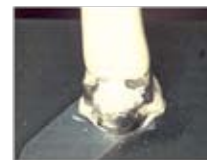
Figure 3-6 Overcrimped leads & wiring at joint
