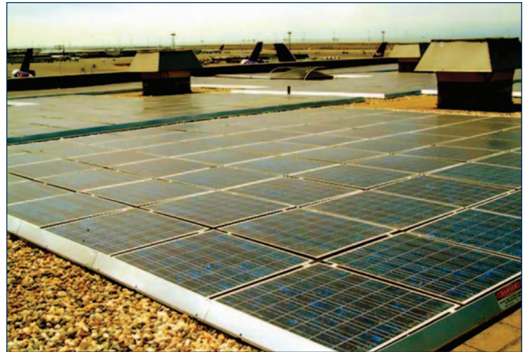
Figure 1-2: A solar array on the roof of a Federal Express hub in Oakland, CA covers 80% of its peak energy needs.
